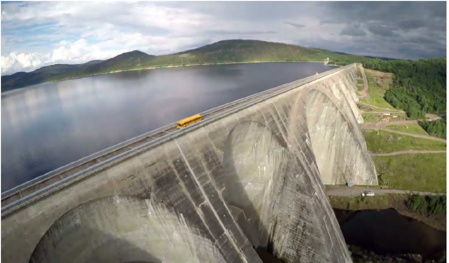
Photo: Hydro Quebec
